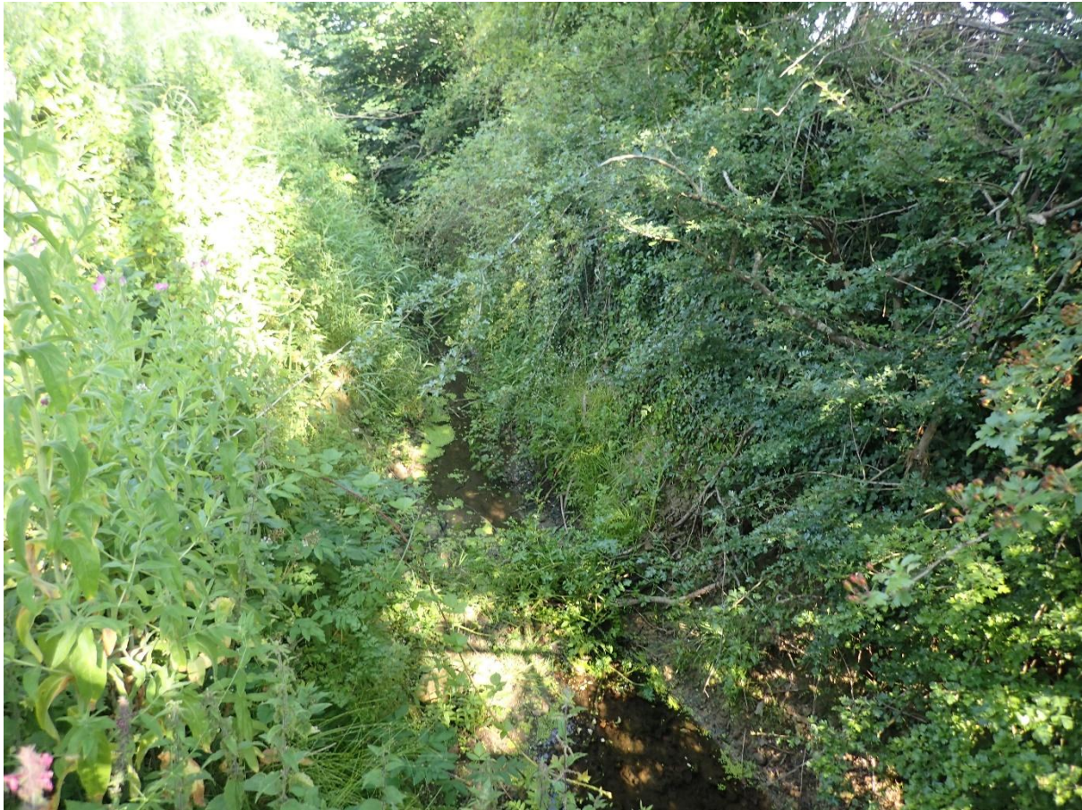
Figure 3-6: Overgrown channel recorded at Site 4 on the Parkroe stream (18/07/2022).
